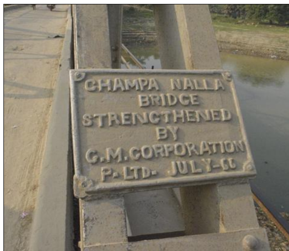
Fig 2: Plaque on the Champa Nalla Bridge, recording strengthening work by "C.M. Corporation P. Ltd." in July 1966. The plaque provides material evidence that the form "Champa Nalla" was publicly used in bridge and infrastructure nomenclature by 1966. Photograph from DainikJagaran series on River Champa
